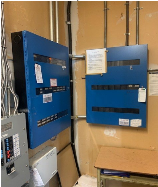
Fire alarm control panel
