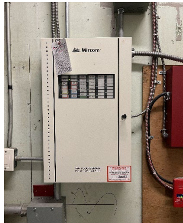
Fire alarm control panel
